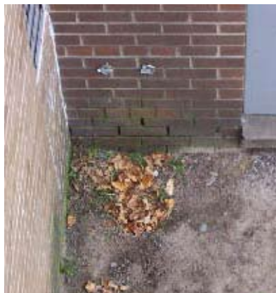
Ponding and Wall Deterioration
